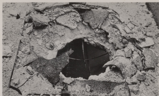
THE HOLE IN THE ROOF OF THE HOSPITAL FOR SICK CHILDREN, GREAT ORMOND STREET, LONDON, W.C.1., CAUSED BY A NAZI H.E. BOMB.
