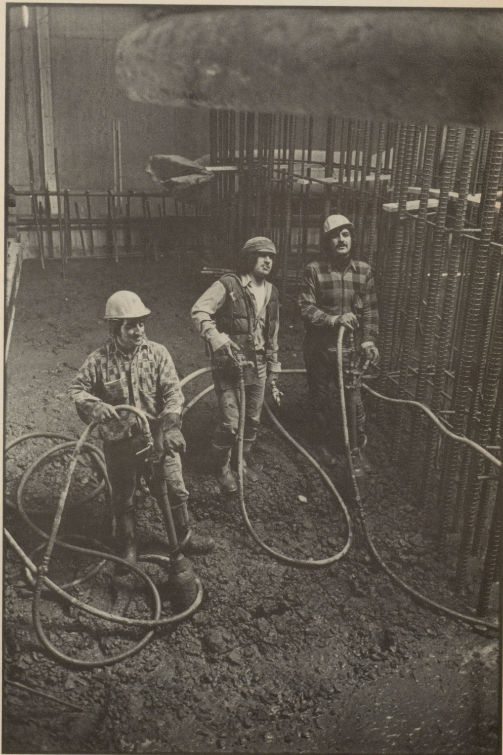
"Concrete crew in power house bay no. 7. The guy in the middle has a bucket-breaker hook-up - he opens the bucket gradually. The other two guys have eighty-five-pound concrete vibrators."
