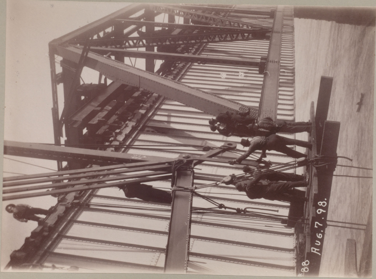
Preparing To Couple Erection Truss With Cantilever Arm — Centre Span Aug 7 th 1898 —
